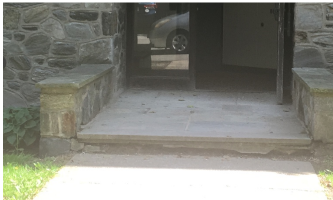
The back entrance to Lunt Hall which could easily be converted to an accessible entrance.
