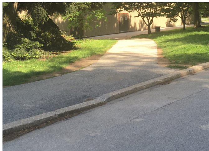
The raised curb which makes the path to the Field House inaccessible.
